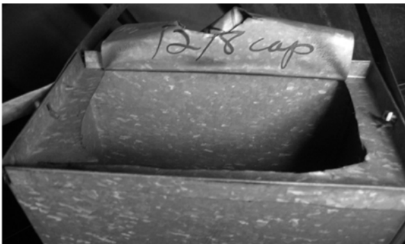
Figure 2: An access point forgot by a duct cleaner allowing 2000 CFM S/A into non-conditioned space.
